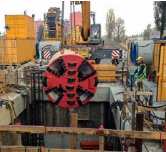
Ablassen der Maschine in den Startschacht Lowering the machine into the entry shaft
