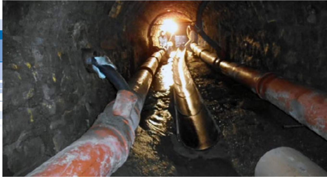
Arbeiten in beengten Verhältnissen stellten sich unsere Mitarbeiter in Gera Our staff in Gera had to complete some of the work in very cramped conditions
